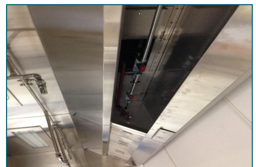
Heat sensitive fusible link valve located in extract plenum which activates suppression system.
